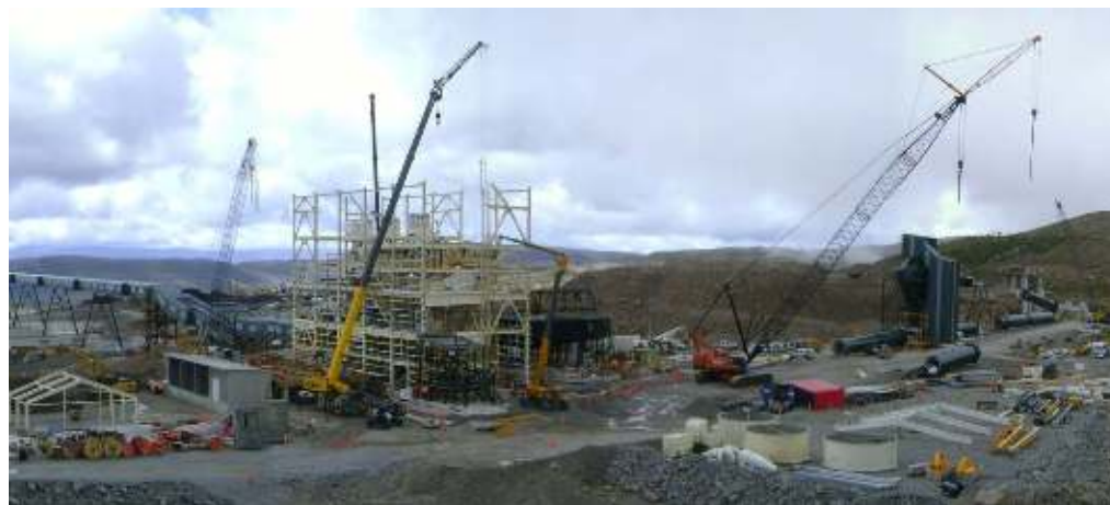
Stockton (New Zealand) Coal Preparation Plant 250 t/h
