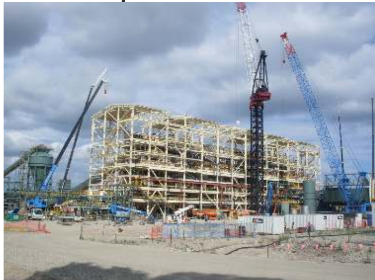
Mangoola (NSW, Australia) Coal Preparation Plant 1800 t/h
